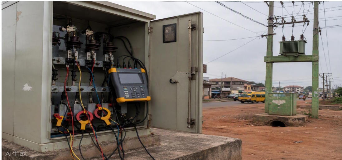
Figure 3: Class-A power quality analyzer with clamp current transformers temporarily installed at a pole-mounted 11 kV ring main unit on the study feeder
